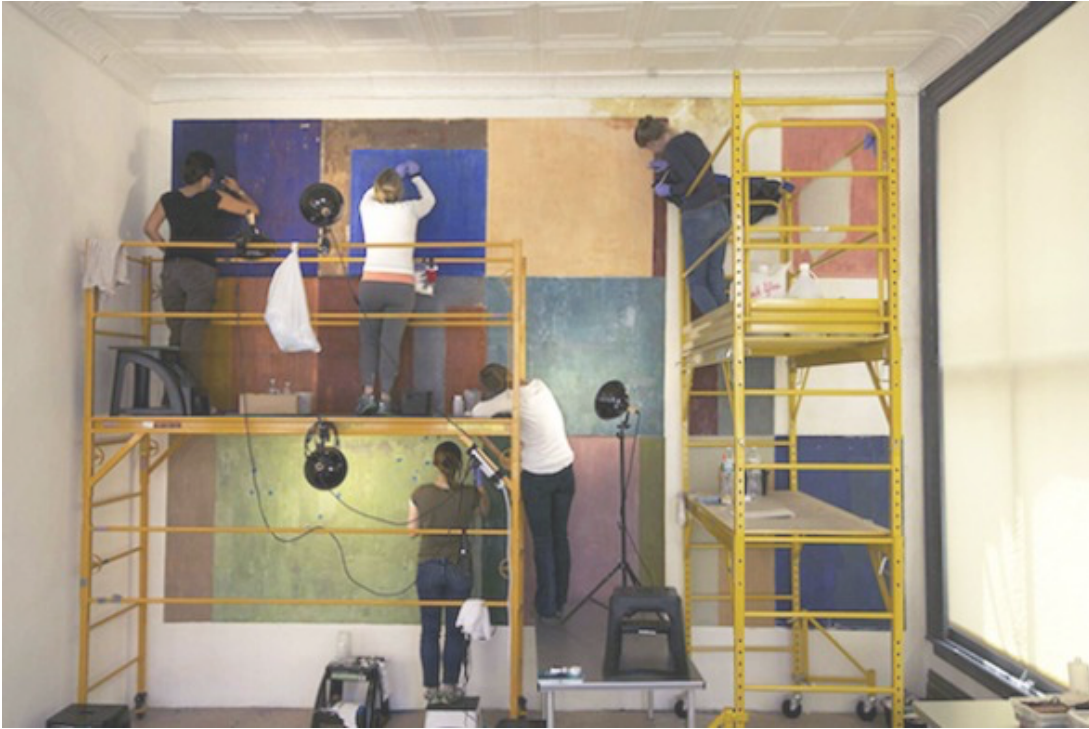
Conservators at work on the treatment of David Novros fresco at Donald Judd's studio, 2014.
